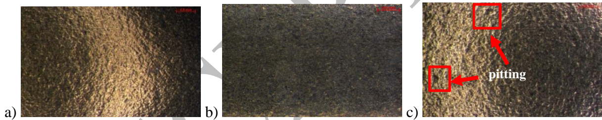
Fig. 17. Examples of corrosion damage on the samples: a) PE, b) PES, c) PESR, mag. 18.9 x
